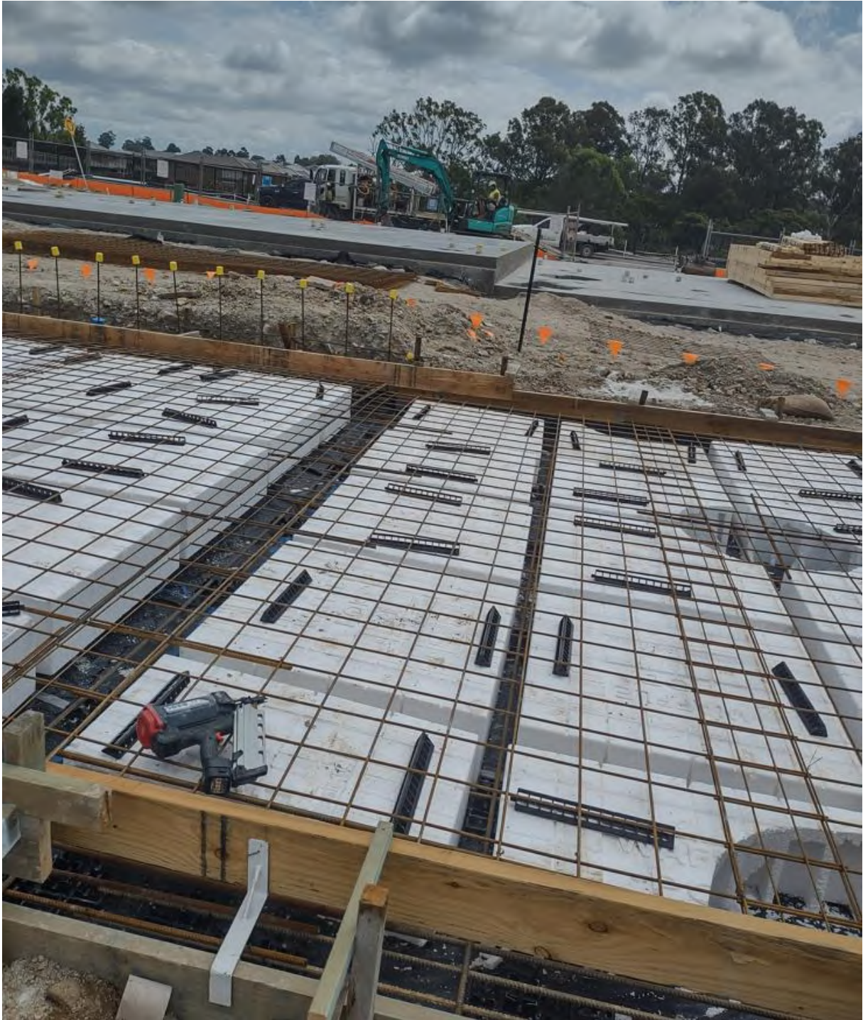
Figure 5: Concrete slab (steel reinforcement and waffle-pods placed over the geotextile, pre-concrete pour)
