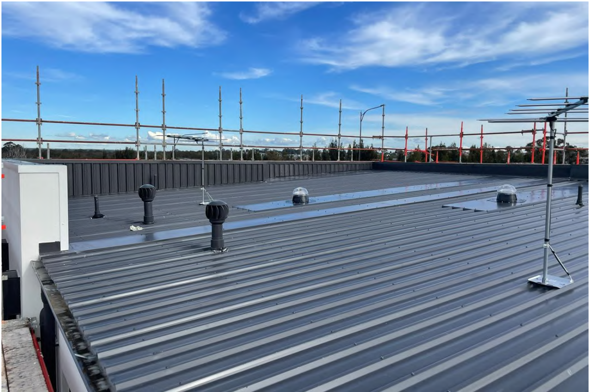
Figure 7: Turbine ventilator (wind-driven) connected to under-slab drainage layer
